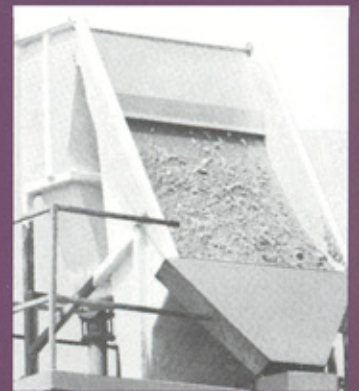
Wastewater Screening For Carrot Processor
