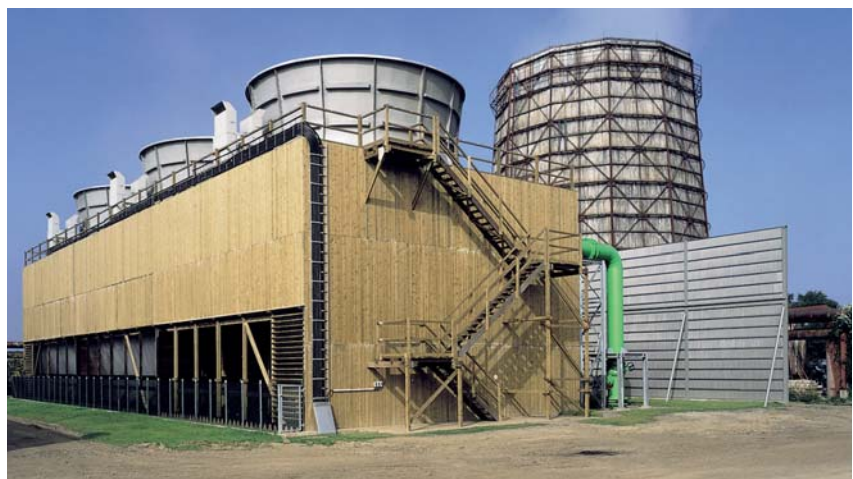
Cell cooling tower with sound attenuation wall
