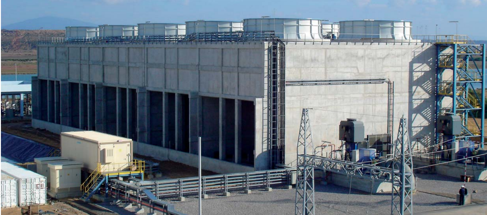
Cell cooling tower (concrete construction)
