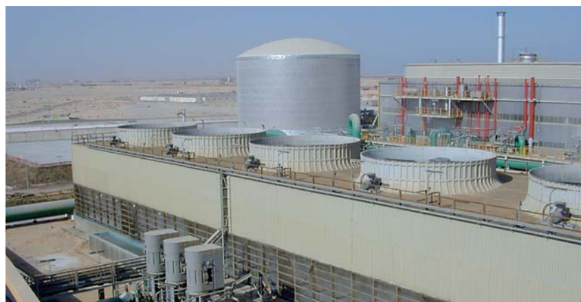
Cell cooling tower (timber construction)
