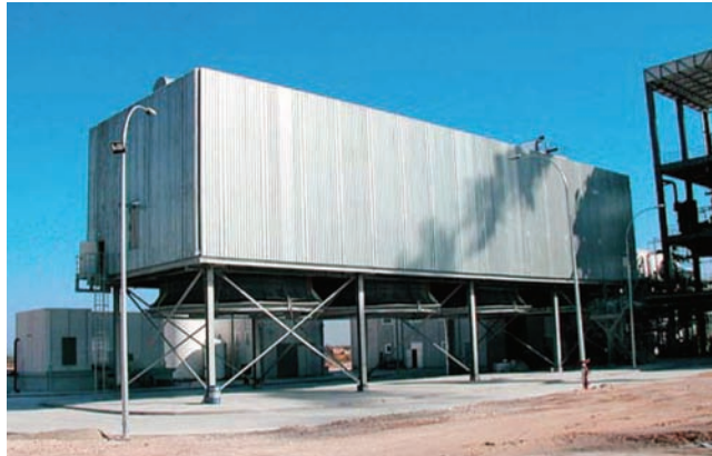
ACCs for 15 MW Power Plant fueled with Dry-Waste Biomass from the Olive-Oil Industry in Spain
