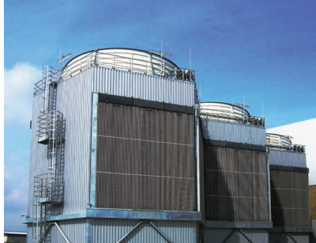
Hexacool for 20MW Biomass Plant in Emichheim, Germany
