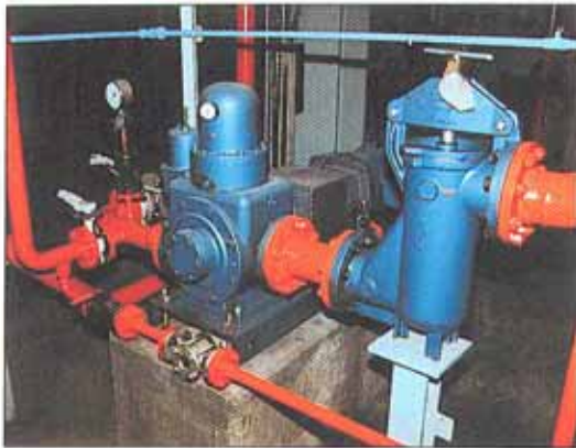
U2000 Pump with Gas Loaded Constant Pressure Control pumping Lube Oil to drum filling machine.
