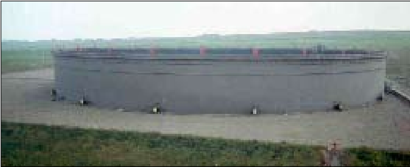
Plenty swivel angle belt drive mixers on a 1,000,000 Bbl (160,000 m 3 ) crude oil tank in Europe.
