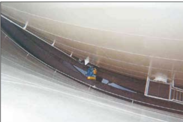
Plenty Mixer installed on a double skinned tank.
