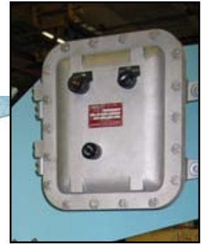
Timer Control Panel
