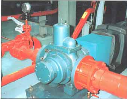
G2000 Lubricants Transfer Pump connected to piping with compressed air purge and pigging system.
