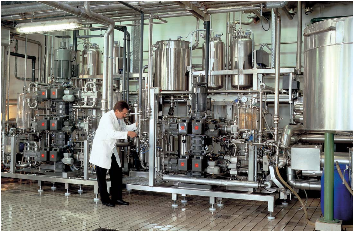
This 16-component installation produces 20 tons of liquid soap per hour. Computer-controlled automation includes recipe management, raw material usage and production reports. Flow monitoring ensures the highest possible accuracy.
