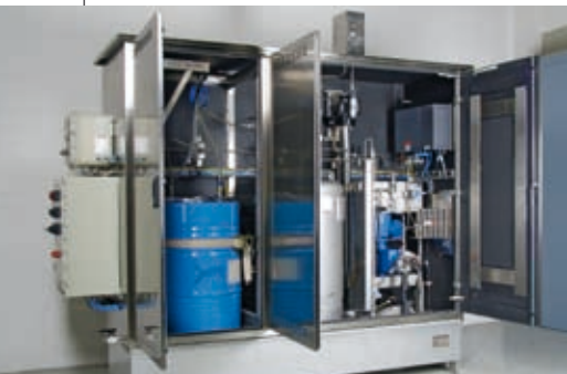
OD 240 in cabinet with 2 x LEWA ecoflow LDB diaphragm pumps and LFM 10 flow meter
