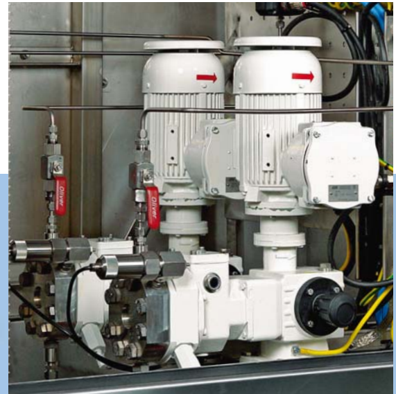
LEWA metering pumps are a practice-proven basic component for odorization systems
