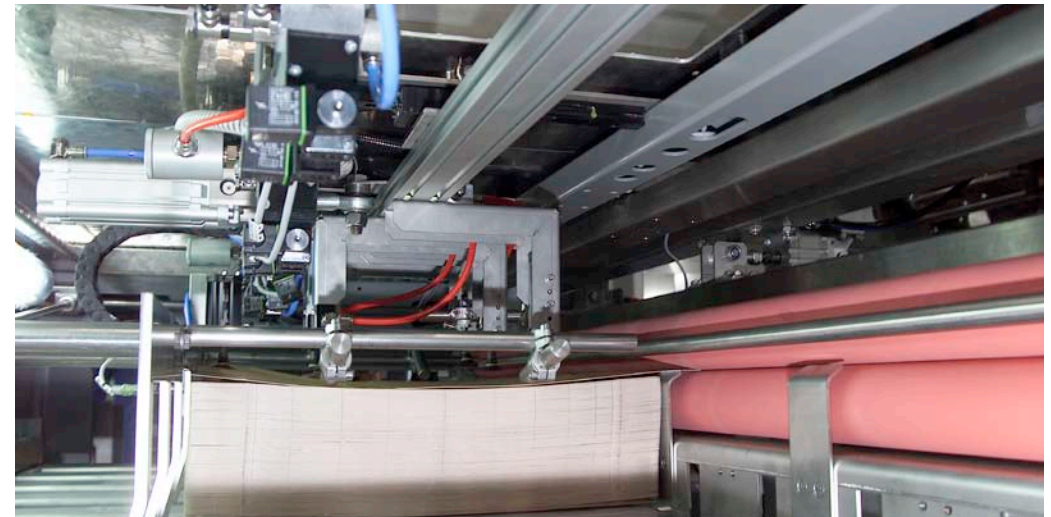
Roller separator feeding the separated cartons.
