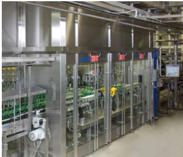
Clean room housing
