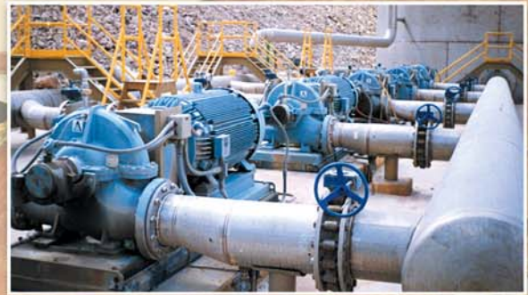
All 316 stainless steel model 3409 pumps on a solvent extraction application at a large copper mine.
