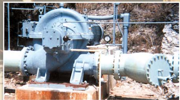
Model 3420 splitcase pump in service at an electric utility plant in the Bahamas.
