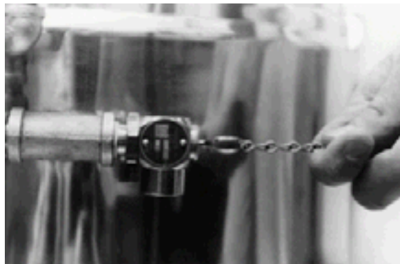
Test the safety valve each day
