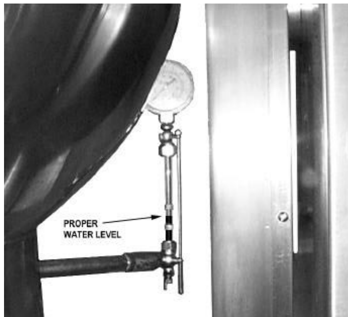
Each day, confirm the jacket water level by checking the water gauge.
