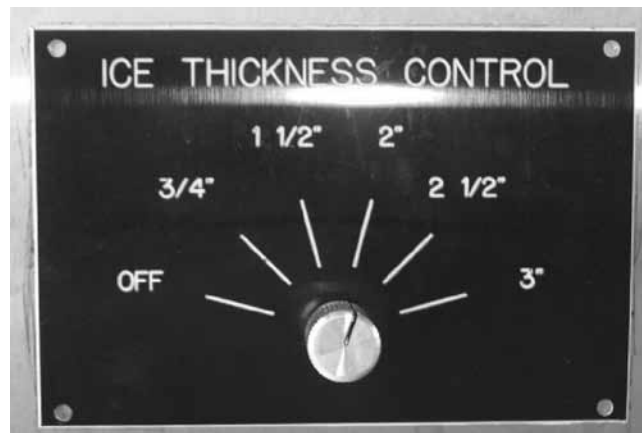
Ice Water Thickness Control Panel
