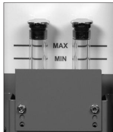
Oil fill level site glass.
