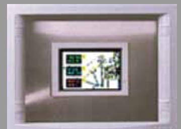
HMI touchscreen controls
