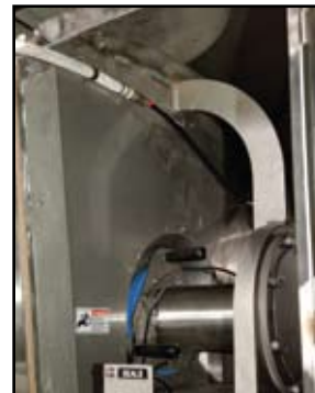
Sanitary Main Shaft Seals
