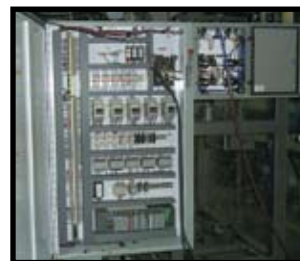
Standard Electrical Panel
