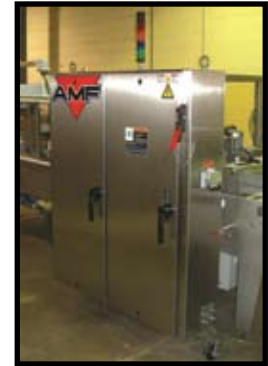
Machine Mounted Electrical Panel
