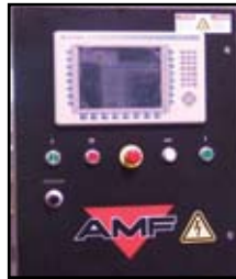
Operator Interface Panel
